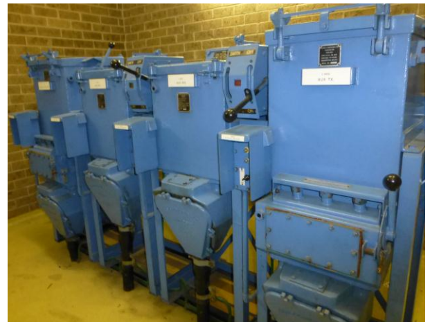
Figure 7. Long & Crawford ETV2 oil auxiliary switchgear (Carramar ZS)
